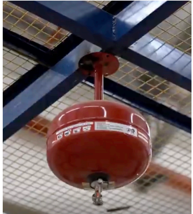
Advanced fire systems
